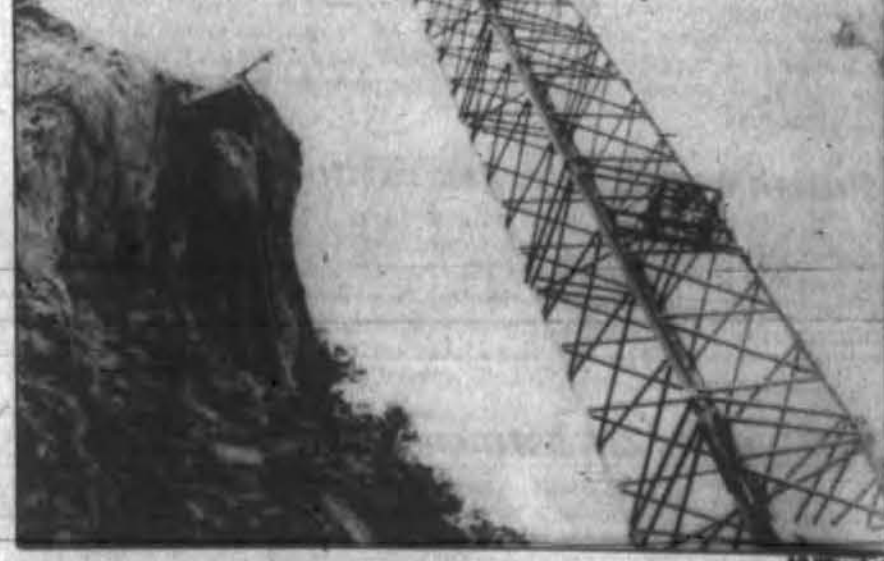
Workers are literally bolting and gluing a mountain together in the Great Smoky Mountains of North Carolina to stop boulders from crashing onto Interstate 40 below.
